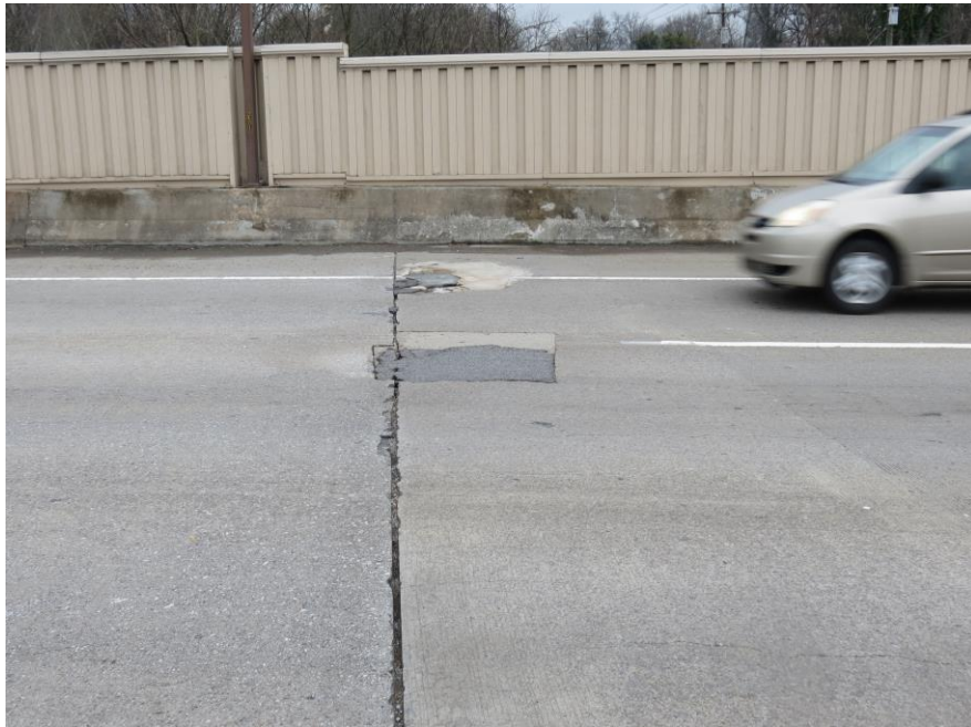
WEARING SURFACE "B" END W/ PATCHES & POTHOLE
