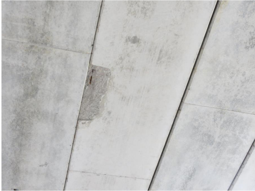
BOX BEAM "H" W/ SPALL & EXP. REBAR
